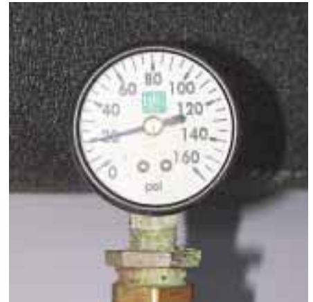
A pressure gauge can show leaks in the loop.
