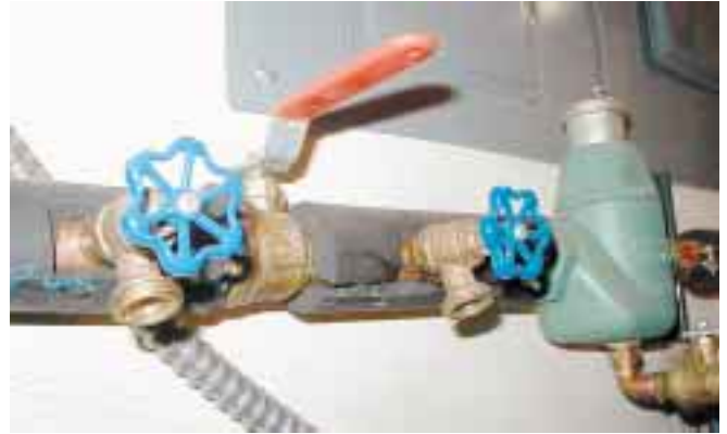
Three valves make up the drain/fill assembly.
