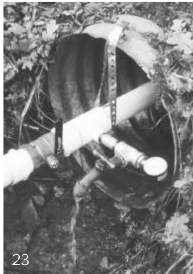
23. The drain valve, inline ball valve, and pressure gauge are clustered together about 10 feet from the hydro unit.
