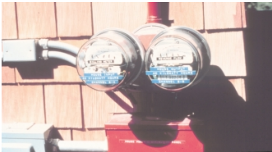
Dual meters are common when renewable energy systems put power back down the utility line.
