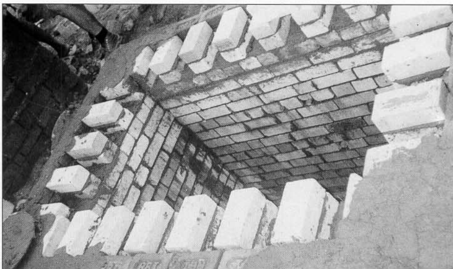
Fig. 2: View showing flue details
